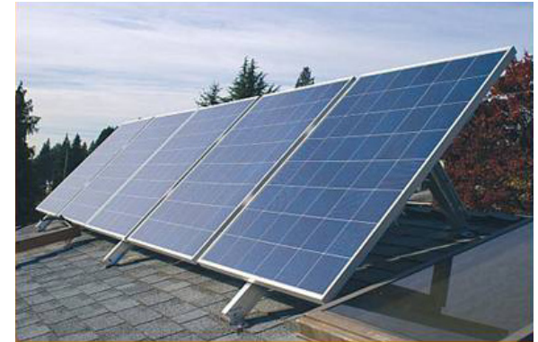
Example of roof mounted photovoltaics panels which generate electricity from the sun's energy.
