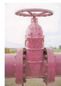
Recycled water pipes are identified by their purple color.
