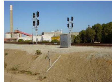
Signals located south of Quint Street Bridge.
