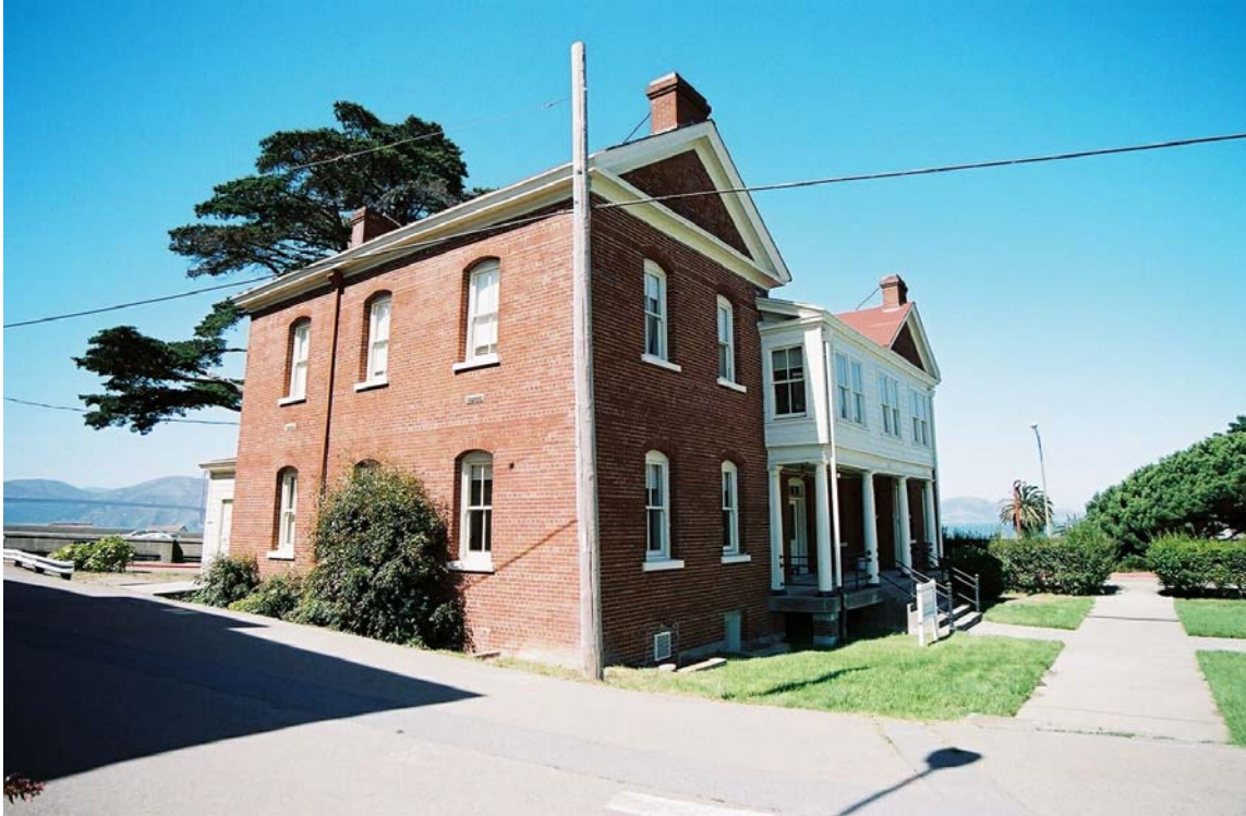
FIGURE 9-6 BUILDING 106 (MAIN POST) SHOWING TYPICAL EXISTING CRACKS IN EXTERIOR WALLS (PHOTOS TAKEN 8/28/04)
