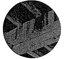
Doyle Drive Structure Degradation
