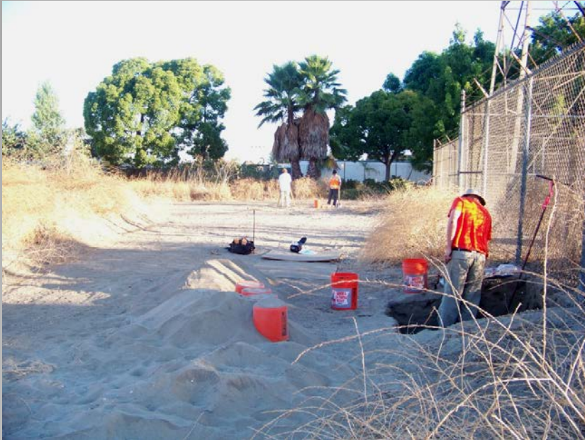
TRTP Transmission Line
