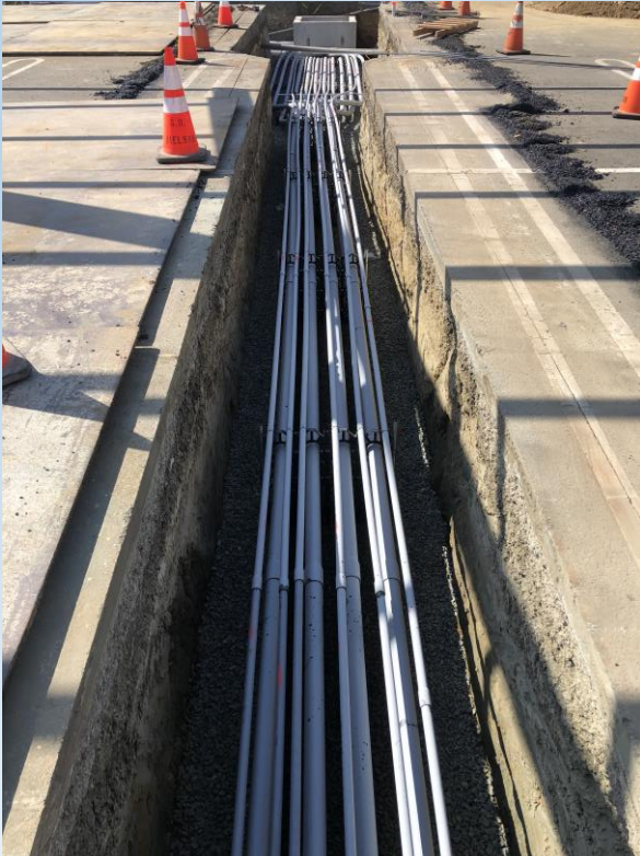
SOLTRANS CURTOLA PARK & RIDE INDUCTIVE CHARGER
