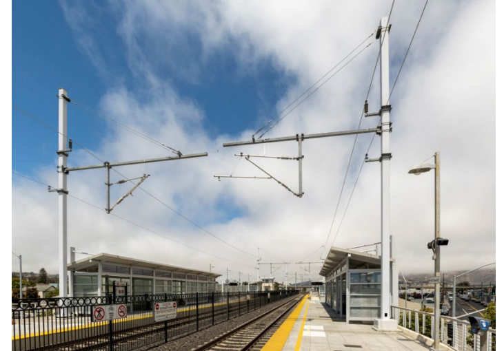
Overhead Catenary System
