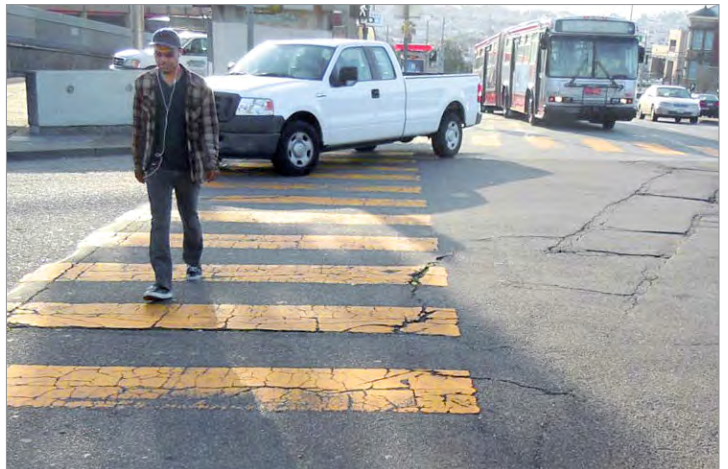
The interchange modifications aim to enhance pedestrian and bicyclist safety by reducing conflicts between I-280-related auto traffic, bus operations, and pedestrian crossings.
