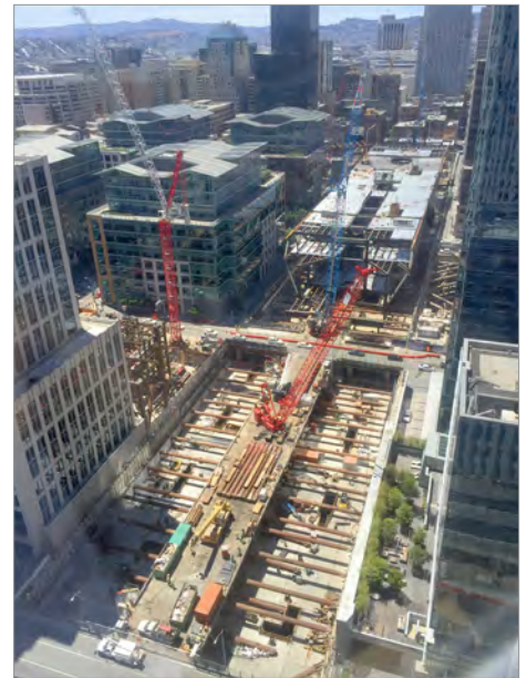
The Transbay Transit Center runs between 2nd and Beale streets. Above-grade construction is now well underway.
