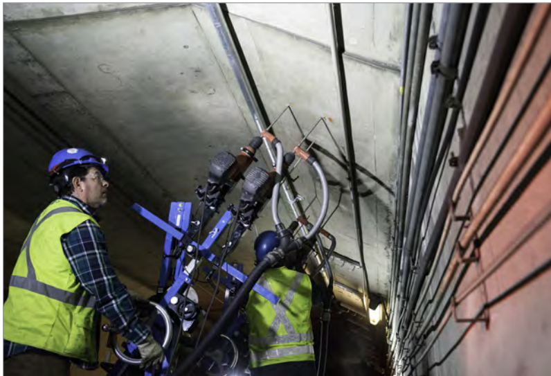
SFMTA's communication infrastructure will be completely updated and expanded. Here, workers install new cable for the subway antenna system in the Twin Peaks Tunnel.
