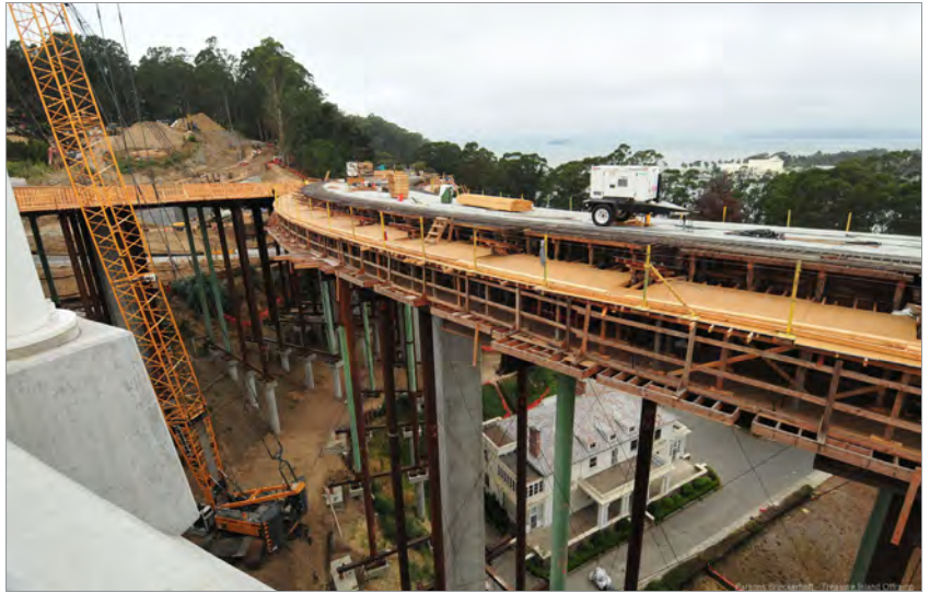
Significant progress has been made, including construction of all foundations and columns and approximately 80% of the bridge decks.
