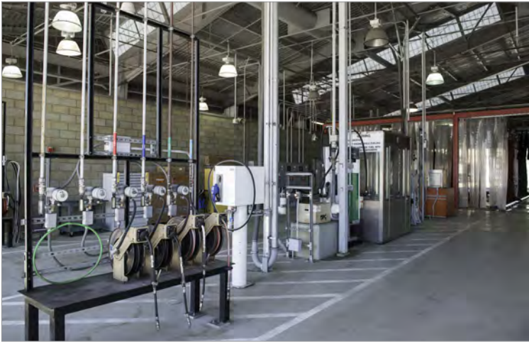
Islais Creek Maintenance Facility is being designed and built to service both 40-foot and 60-foot articulated motor coaches and will be able to support maintenance of the Van Ness BRT fleet.
