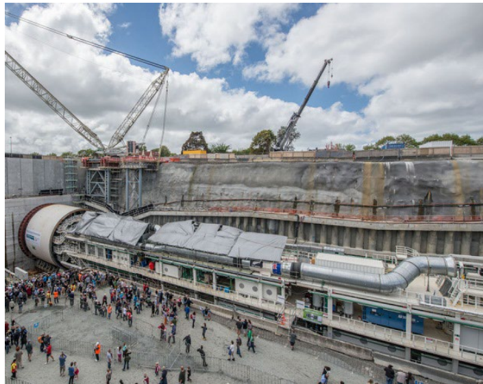
Figure 7-7. Example of a TBM Set Up and Ready to Excavate into a Headwall (46-foot-diameter TBM, Waterview, NZ)
