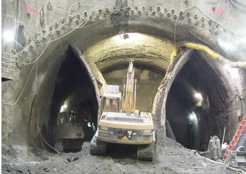
Figure 7-2. SEM Construction Example, Showing Pipe Support Over Tunnel Crown and Sequentially Excavated Tunnel Drifts (Beacon Hill Station, Sound Transit, Seattle)
