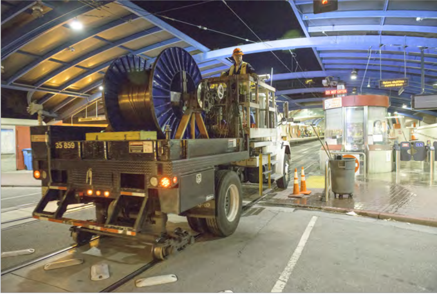
SFMTA radio replacement work is entering the final phases. Here, a Line Dept. vehicle enters the tunnel at West Portal. ▲
