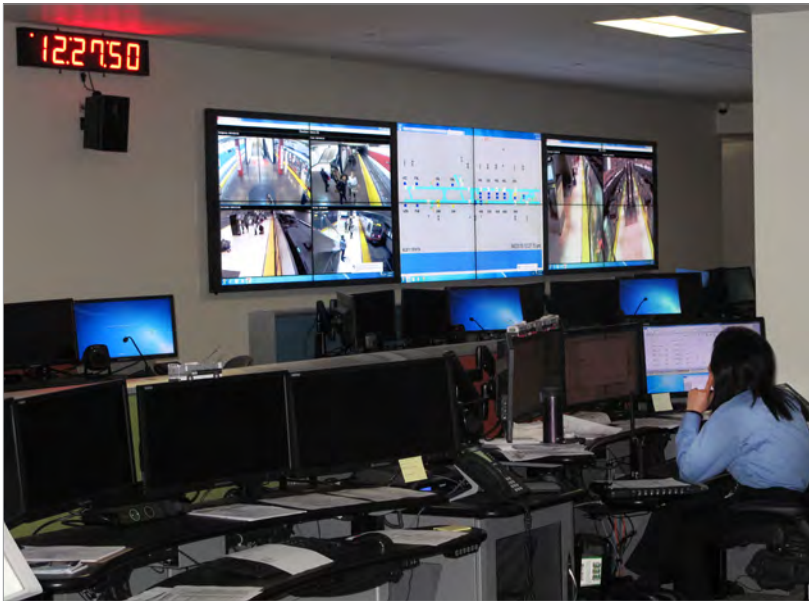
Prop K funding is helping SFMTA expand its control and communications functions at its new C3 Center. ▲
